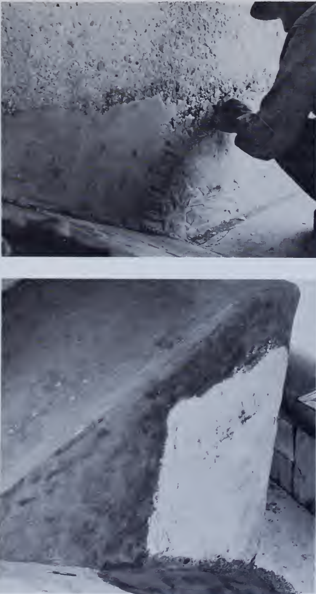
Figure 184.—Epoxy-bonded epoxy mortar repairs. In upper photograph epoxy mortar is placed on epoxy bond-coat previously applied to wall of sluiceway at Yellowtail Afterbay Dam. The lower photograph shows a dentate in sluiceway repaired with epoxy-bonded epoxy mortar. The difference in mortar color in the two photographs is caused by use of different colored sands. P459-D-68911 (upper), P459-D-68912 (lower).
